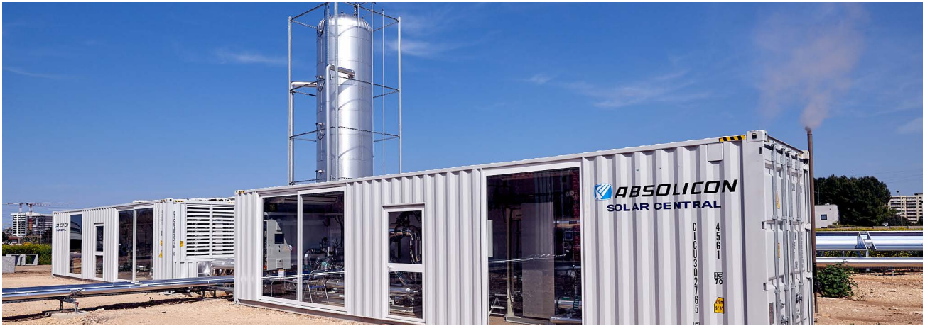
Hot water storage tank and solar central at the Birra Peroni brewery in Bari, Italy. Credit: Antonio Tartaglione
