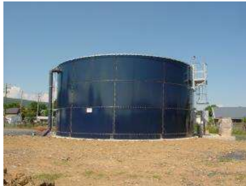
Tank thermal energy storage (TTES) (60 to 80 kWh/m 3 )
